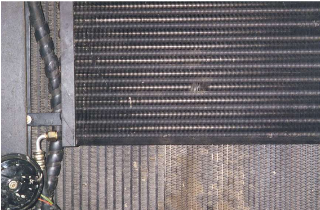
Lower area of condenser showing hose routing.
